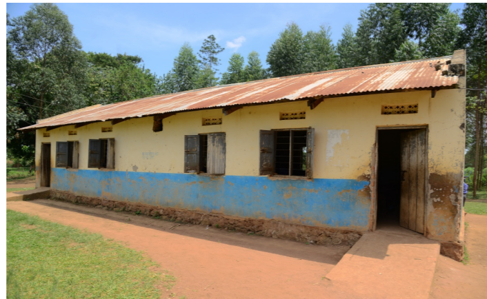
An empty structure of the dilapidated classroom at Karongo Primary School in Kasese, which NSSF is renovating to improve students' learning conditions
